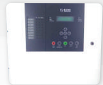
Master Control Fire Alarm
