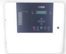
Master Control Fire Alarm
