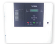
Master Control Fire Alarm
