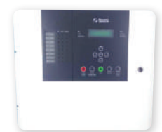
Master Control Fire Alarm
